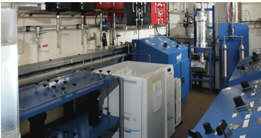
Fig. 5.6 Air fuel synthesis plant for producing 1 ton per day of fuel (reproduced with kind permission of Air Fuel Synthesis Ltd)
