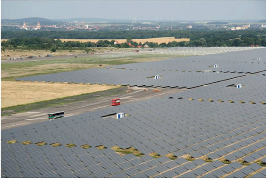
Fig. 4.1 The first solar 40 MW photovoltaic array installed in Waldpolenz, Germany (Photo courtesy of JUWI Group)
