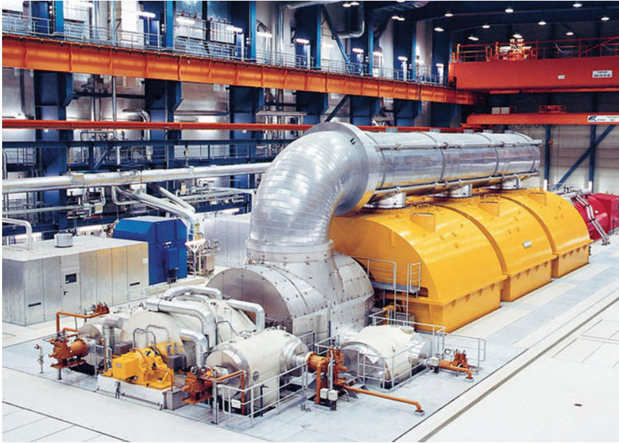
Fig. 2.7 Gas turbine generator (Source http://en.wikipedia.org/wiki/Electricity_generation#Turbines )
