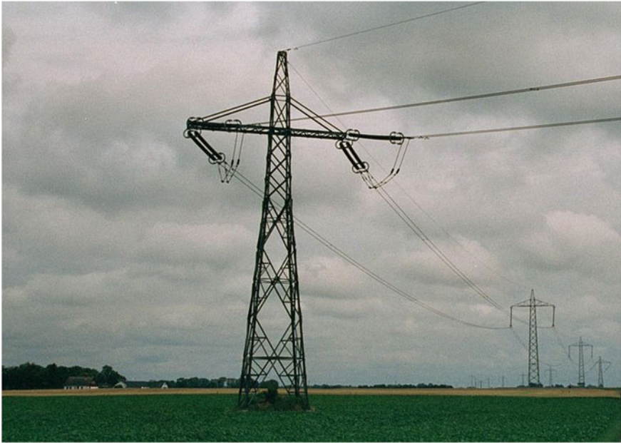
Fig. 3.1 Pylons of the Baltic Cable HVDC in Sweden (Source http://en.wikipedia.org/wiki/High-voltage_direct_current )
