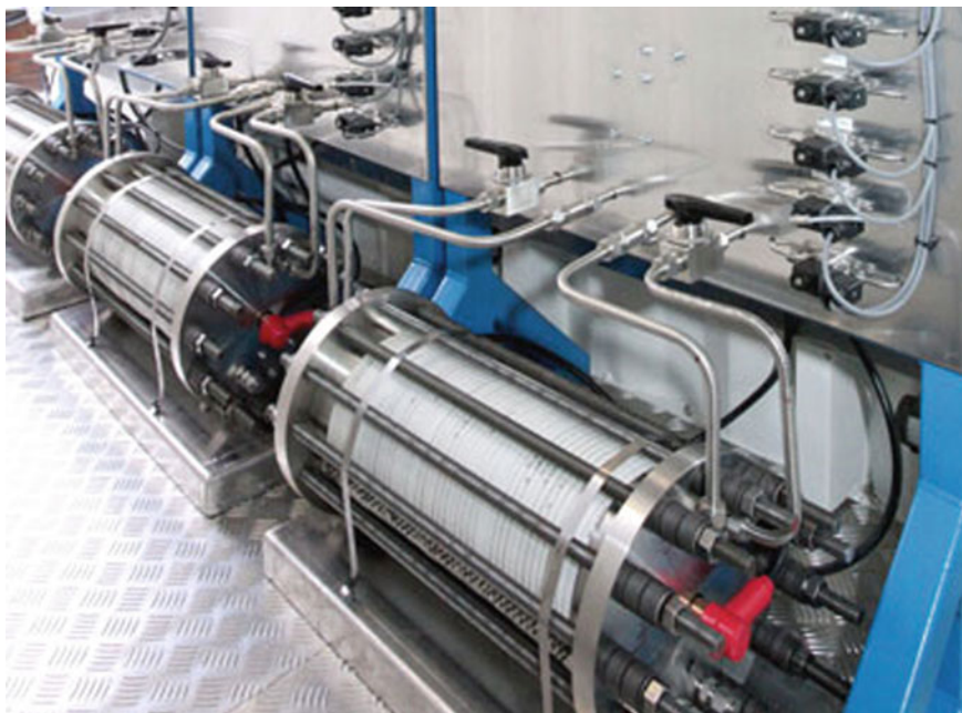
Fig. 5.5 ITM modular electrolysis units (reproduced with kind permission of ITM)
